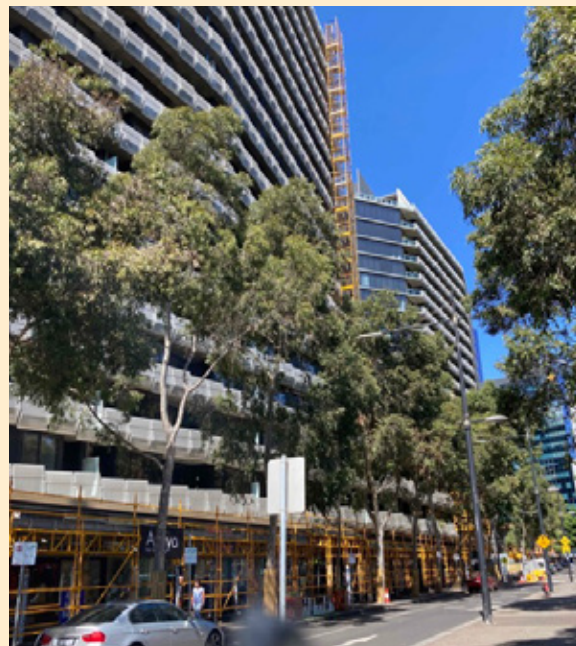
Image: A gantry installed in front of the building in Example 2 well before work commenced, obstructing shopfront visibility and impacting local businesses.
