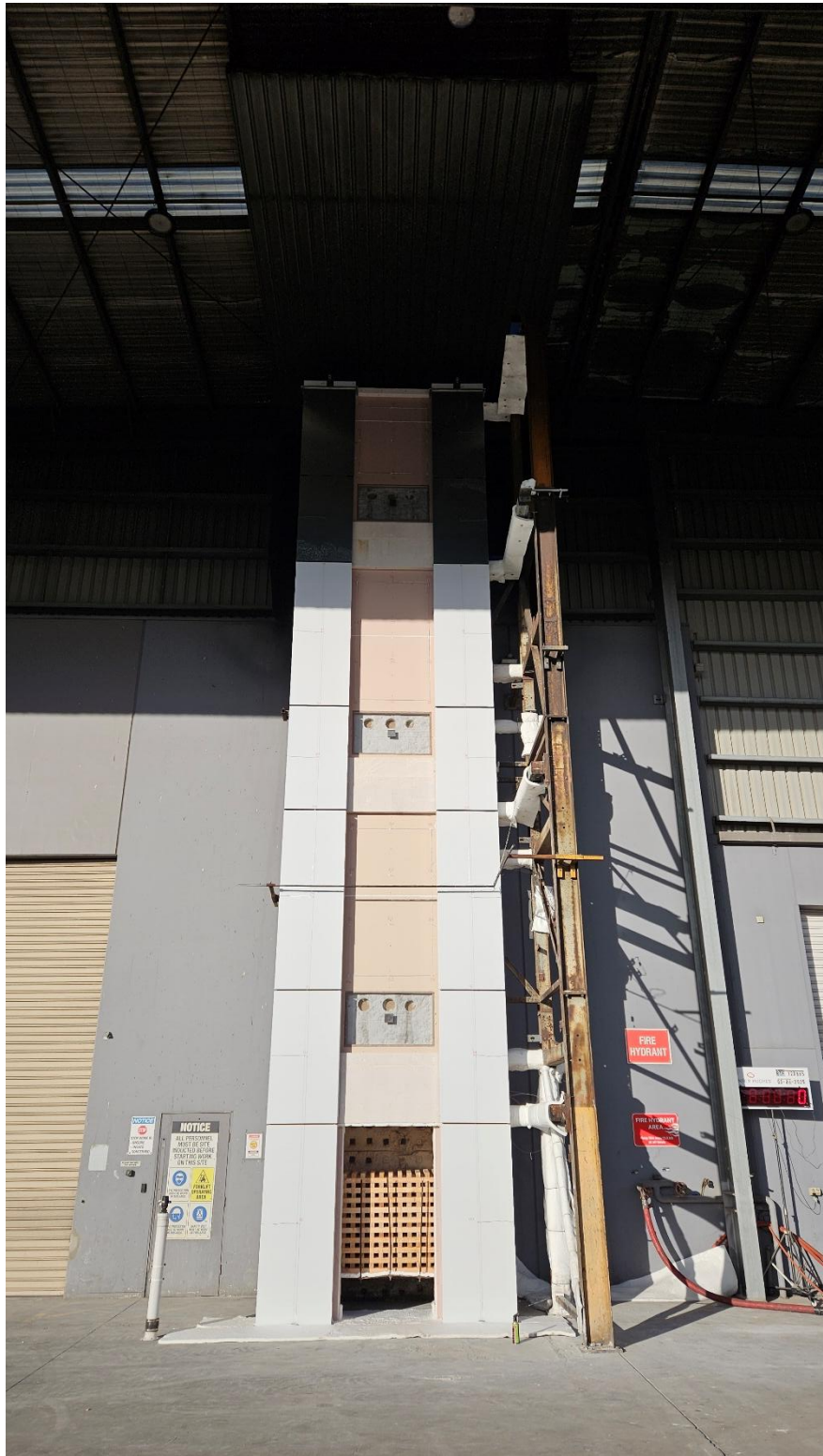
Figure 44 The external cladding system before the start of the test – main wall
