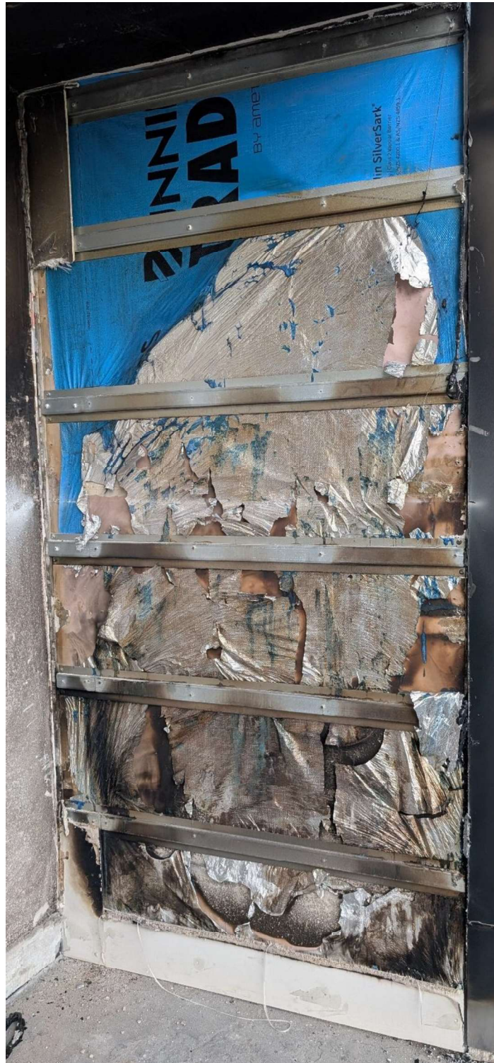
Figure 46 Post test condition behind the MgO board.
