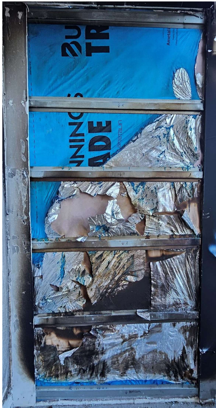
Figure 46 Post test condition behind the MgO board.
