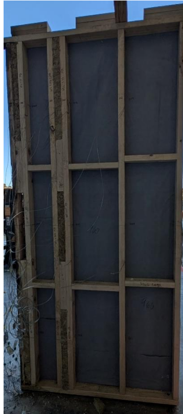
Figure 55 The wall system on completion of the test – behind AAC with insulation removed
