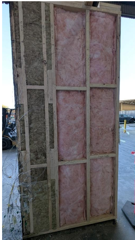
Figure 54 The wall system on completion of the test – behind AAC with plasterboard removed
