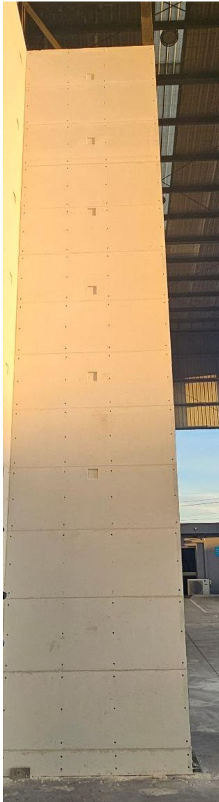
Figure 19 The external cladding system before the start of the test – wing wall
