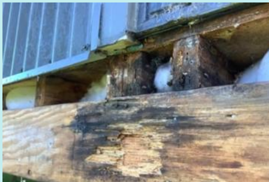
Bearers and joists rotted. No flashing on windows or walls
