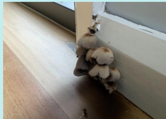
Mushrooms growing on the skirting boards inside the house.
